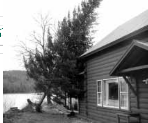
Wind damage from an early Spring storm
